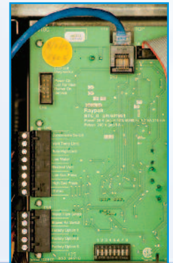
Low Voltage Wiring Center
